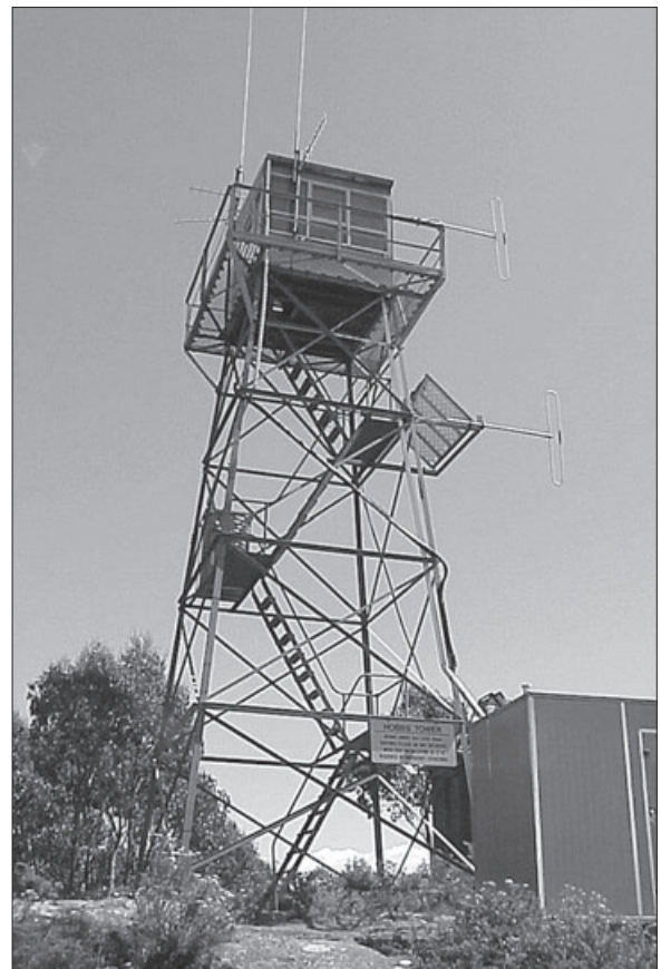
A modern fire tower at Mount Hobbs near Buckland. Note the telecommunications equipment.
