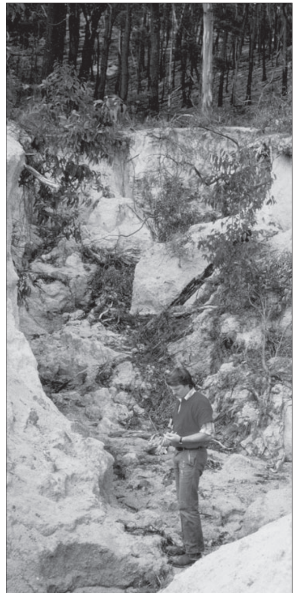
Severe erosion of unconsolidated granite soils in north-eastern Tasmania. (John Grant pictured.)
