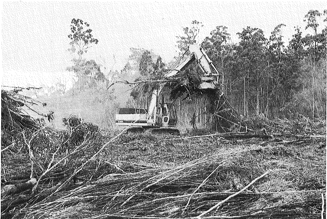
Photo 1. The 30-tonne excavator (above) raking and (below) stacking slash at Esperance BX, with a six-pronged finger raker and thumb grab.
